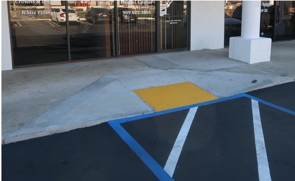
Figure 27. Ramp on the curb of the sidewalk next to a handicapped parking space
