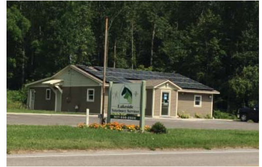
Lakeside Veterinarian Services Solar Installation
